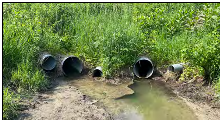
Left to Right: 15", 24", 12", 21", 8" dia. corrugated metal pipe (CMP)
