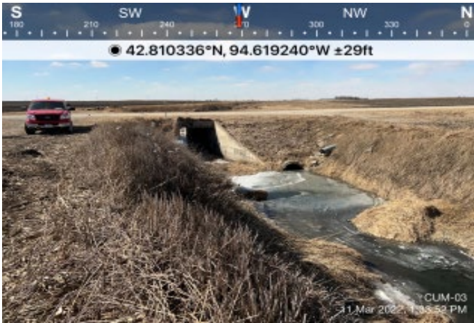
Cut 3.4' needs to be removed and sloughs removed.
